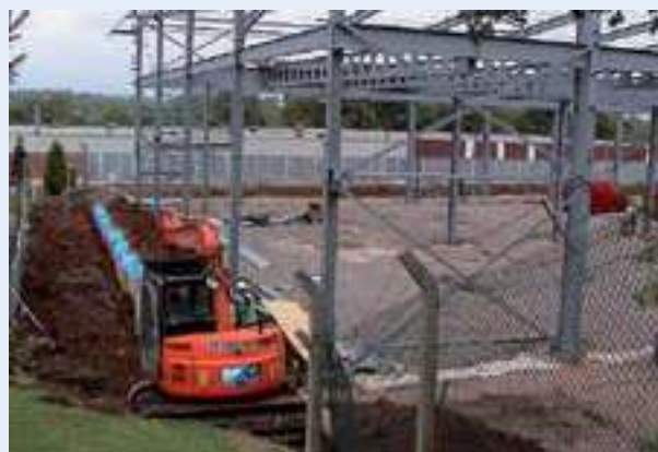
Stage 4: Make sure that the presence of the root barrier membrane is recorded and is not disrupted by future developments and landscaping.
