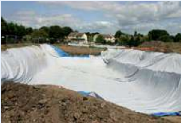
Stage 3: Put root barrier membrane in place, allowing enough material along the edges to eventually provide a seal.
